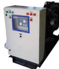
AMF panel mounted on genset
